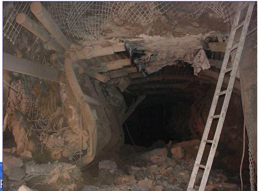
Collapse of a production gallery in the Cullinan diamond mine in RSA (700 m depth)
